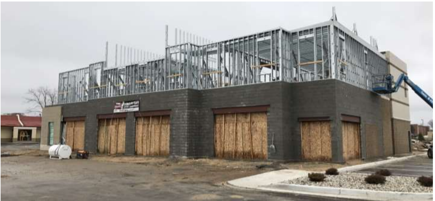
Campus Commons mixed-use development under construction at 1720 S. Mission at the intersection with the newly opened Central Drive.
